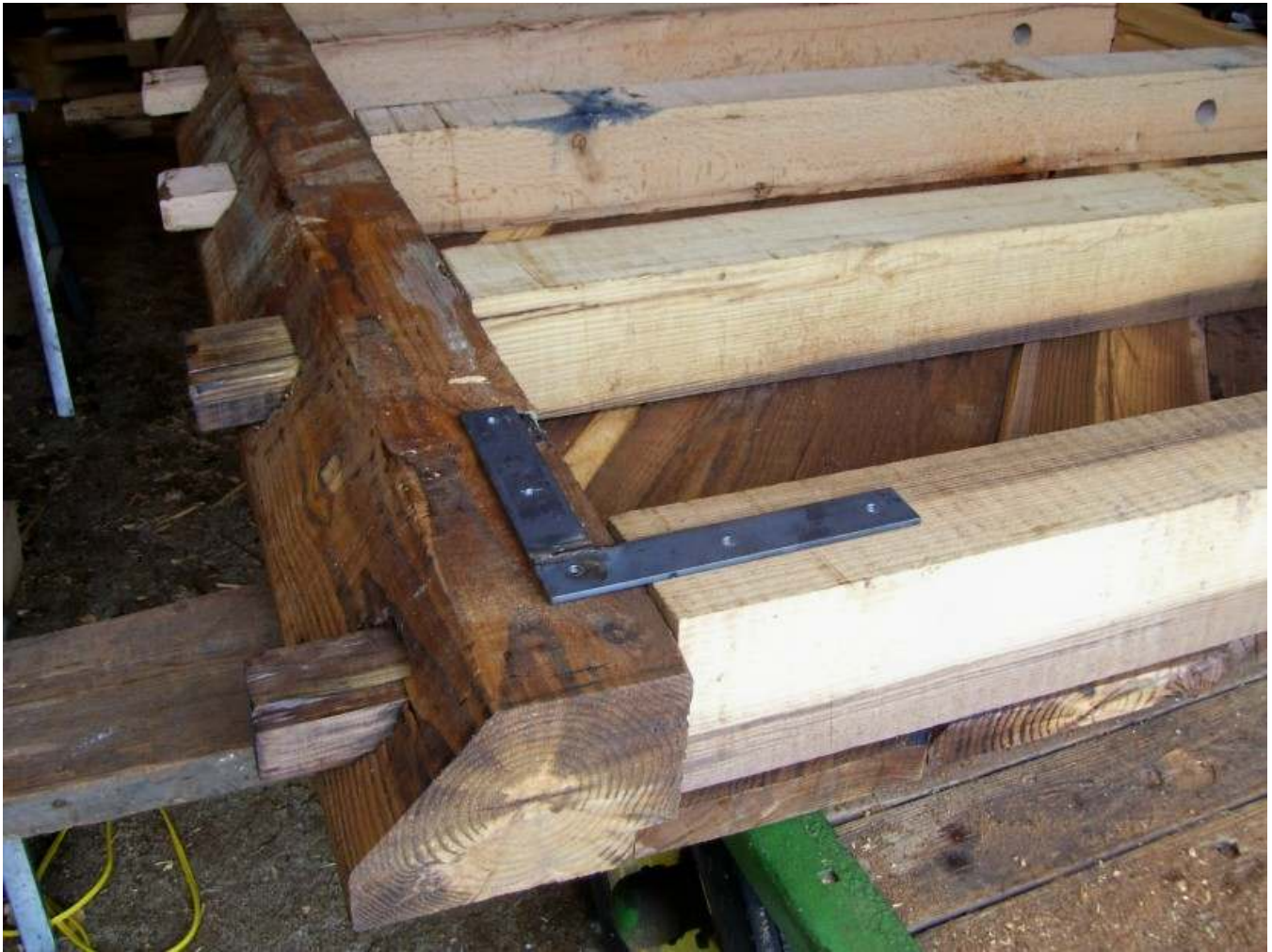
After flipping the gate mortise joints need trimmed and angle brackets installed on that side.
