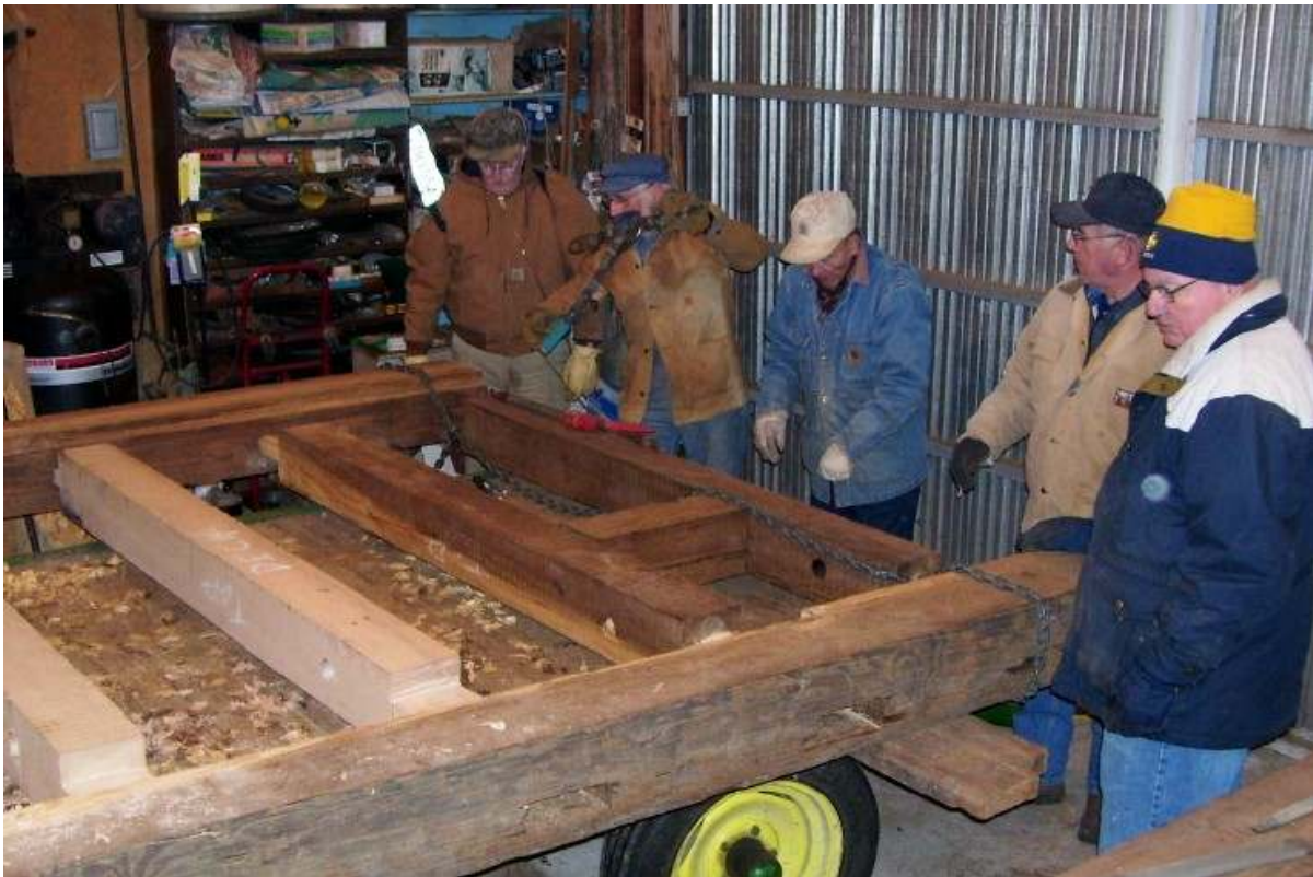
The guys winch the lock gate posts and horizontal timbers together for a snug fit.
