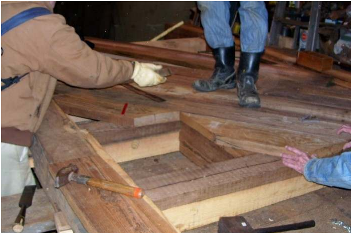
Decking the gate calls for leaving an 18 inch square opening for the metal wicket (water flow valve).
