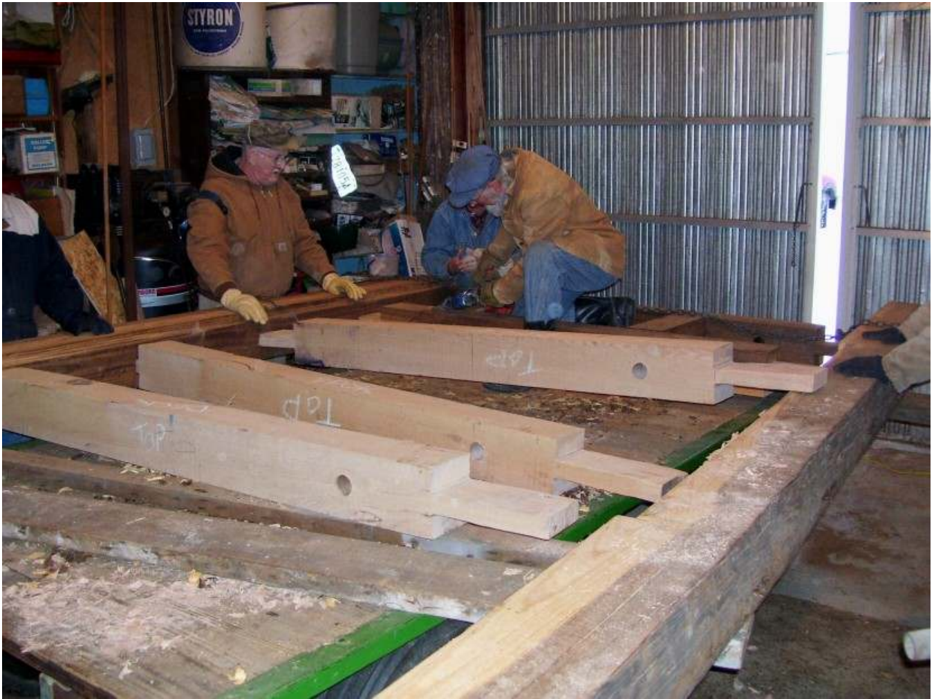
Previously cut mortise and tenons on lock beams are ready for assembly by the volunteer crew.
