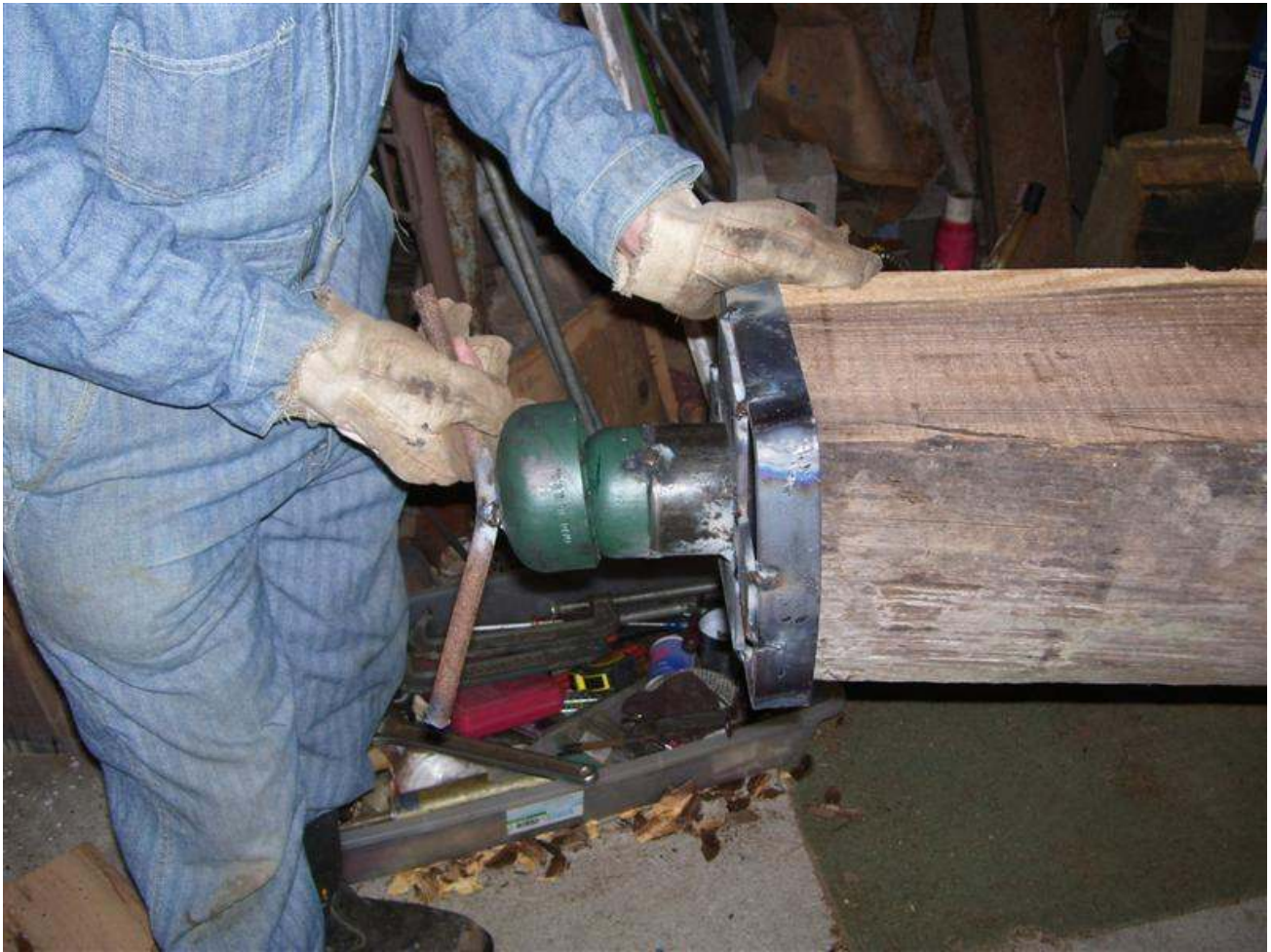
Roy creates the metal bearing called a "GUDGEON" that allows the lock post (laying on its side) to pivot.
