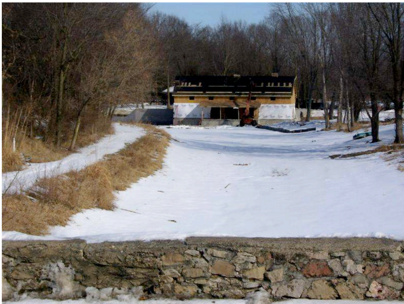
Rising out of the banks of the original "turning basin" north of the Stone Arch Bridge this large building will house the new replica canal boat. The canal is currently drained to allow construction.
