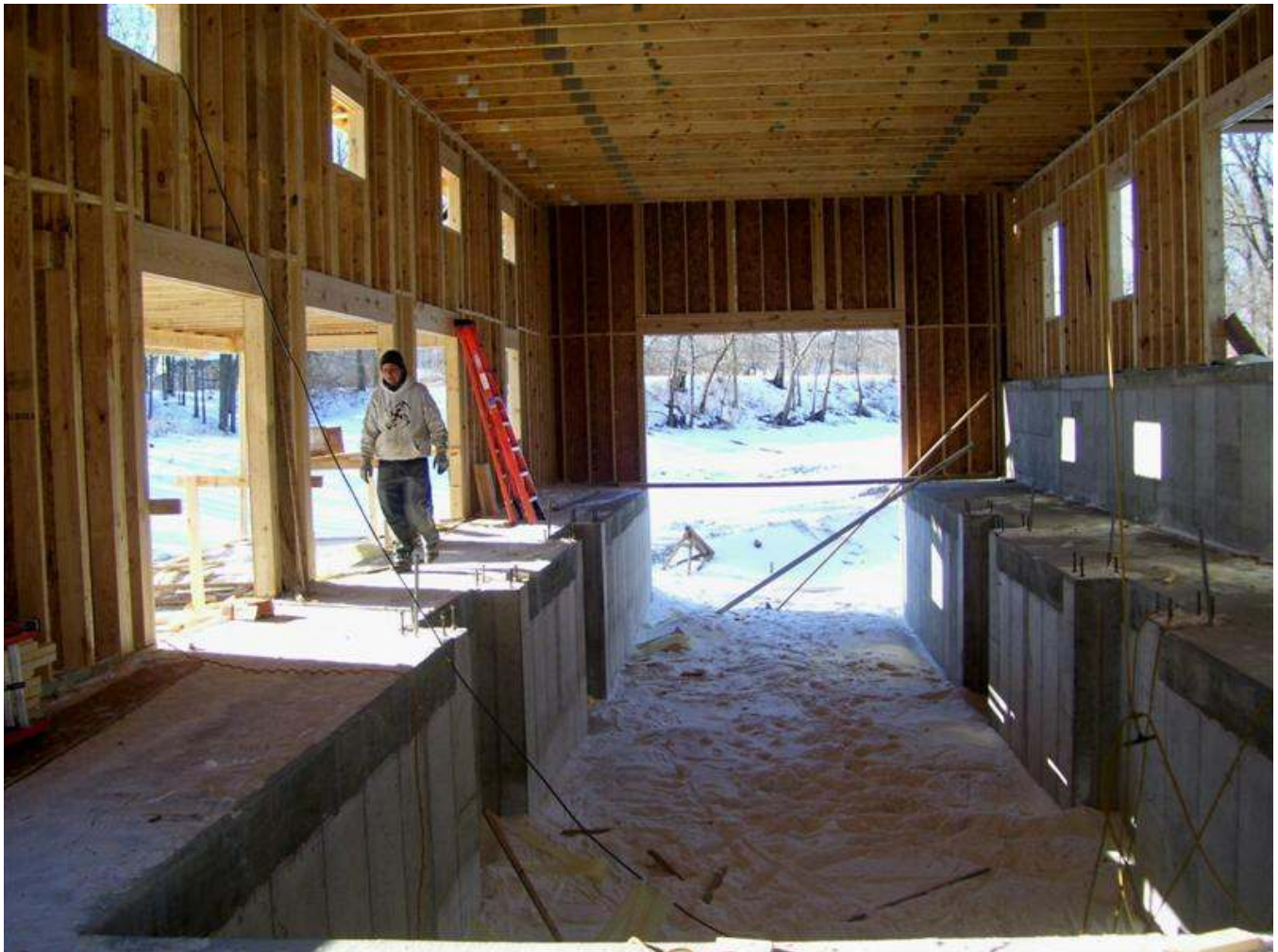
This "slip" (dry today because the canal is drained) inside the warehouse will safely store the new boat. It will allow raising the boat above the water level in winter to protect the hull from ice damage.
