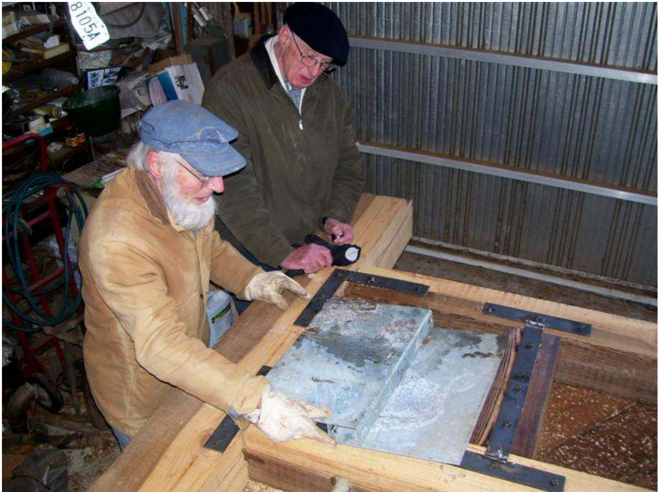
Volunteers Roy Patrick from Lafayette and Ron Dust, our volunteer "Engineer" that comes from Chicago, review the placement and operation of the pivot wicket that controls water flow through the gate.
