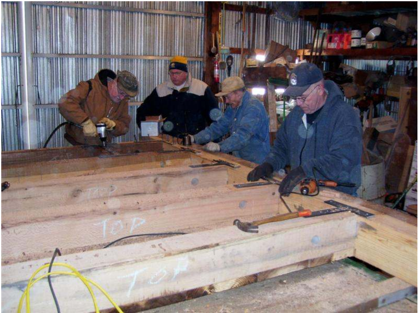
Angle iron braces are being placed on the second Guard Lock gate by the M-W-F Volunteers
